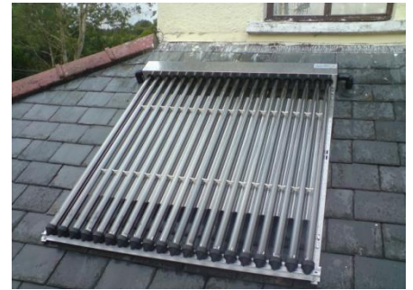
Ted's domestic evacuated tube installation
